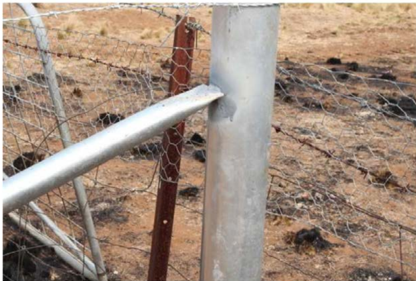
D021 Photo from Kevin Pearce - Strainer post that has been welded at the origin area
